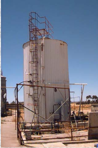
Continuous Flow Stirred Tank Digester at Roseworthy Campus.
