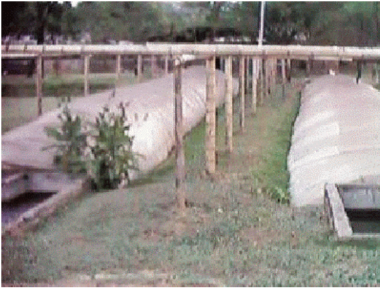
Fig 5 "Poly" plug flow digester
