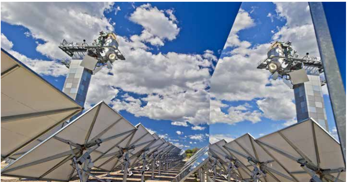
ASTRI Solar Tower (photo courtesy of CSIRO)
