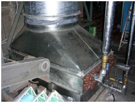
MSS LAS Level 6, Conventional HVAC Heat Recovery Coil – Exhaust Discharge
