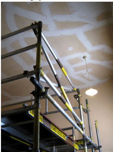
Left: Repairs made to the badly cracked eastern ceiling
