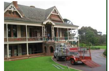
Investigating the falling damp on the northern balcony
